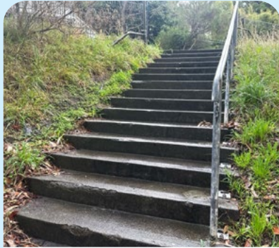
Stair-nosing luminance contrast strip has not been provided. Compliance handrails have not been provided on both sides of the stairway. FTG
