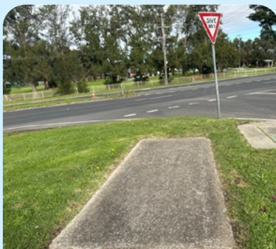
Footpath terminates and does not connect to anything. KF
