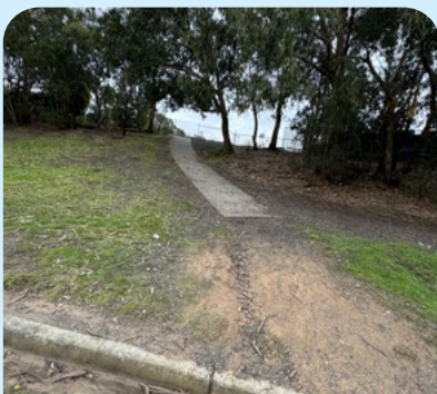
Footpath not continuous. RCC
