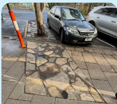
Change in surfaces causes a potential tripping hazard. TBT
