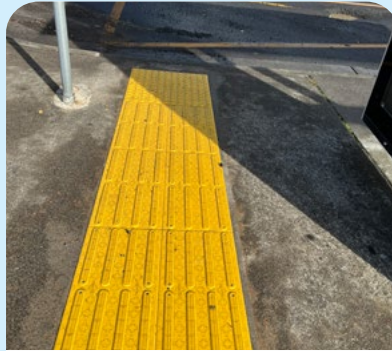
TGSI tactile marker colour contrasts with footpath surface. TBT
