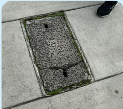
Poorly maintained asset infrastructure causes tripping hazard. SV
