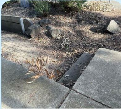
Stair-nosing luminance contrast strip has not been provided. RCC
