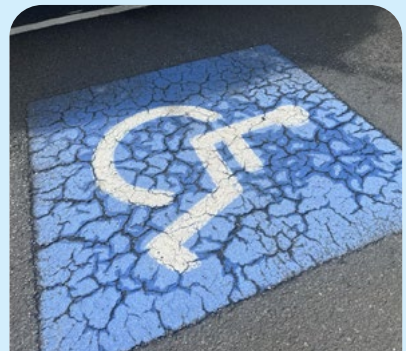
Line markings are broken, faded or have sections missing. FTG
