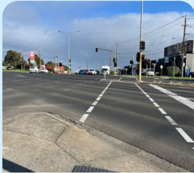
TGSI tactile marker is well maintained, contrasts with footpath surface and angled towards direction of travel. WM
