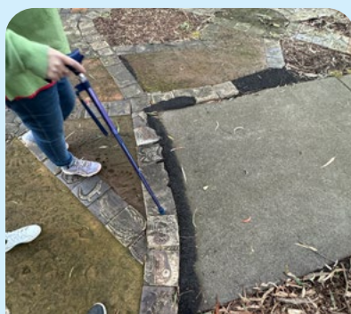
Uneven surface with debris. RCC
