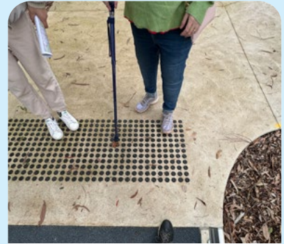
TGSI tactile marker good quality and high contrast with footpath surface. RCC
