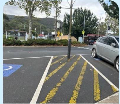
Bollard does not have adequate luminance contrast painting. FT
