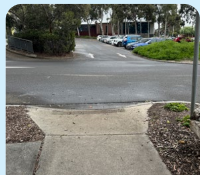
Footpath leads into roadway and does not connect with another footpath. RCC
