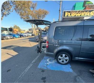
Accessible car park too short, therefore PMDs have to enter and exit the car in the roadway. KF
