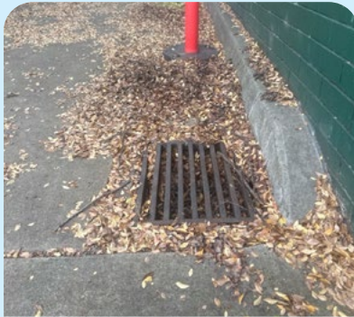
Grated slotted openings are in the same direction as the dominant direction of travel, thus they are a tripping hazard. KF
