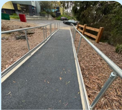
Path surface good quality. And has edges and arm rests. Connects to car park. RCC
