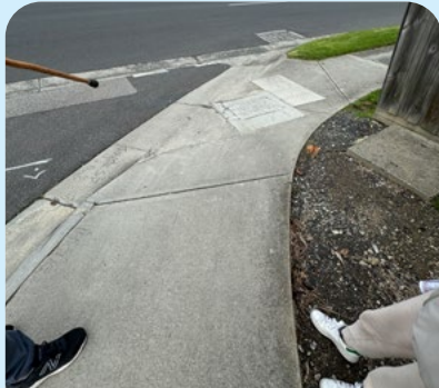
Sloping narrow footpath with curve makes it difficult to navigate. SV
