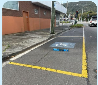
On-street parallel parking end bay is not long enough. FTG
