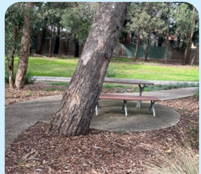
Insufficient space on the concrete pad and under the picnic table to park a wheelchair. RCC
