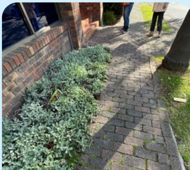
Uneven footpath surface and narrow footpath presents as a tripping hazard. WM
