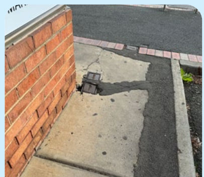
Uneven surface on sloping footpath is a potential tripping hazard. SV
