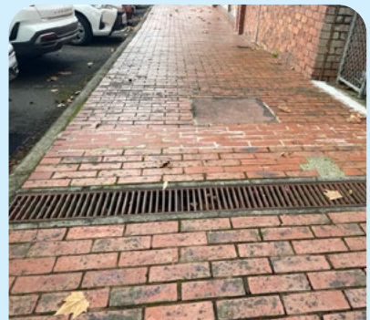
Grate slotted openings are in the same direction as the dominant direction of travel. FTG
