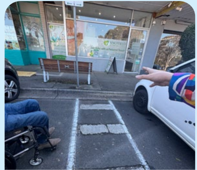
Shared zone too narrow and does not have painted yellow lines. KF
