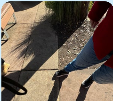
Footpath edge higher, therefore presents as a tripping hazard. WM
