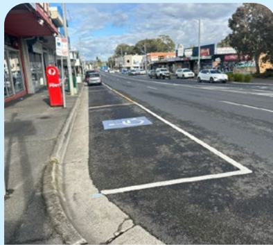
Required kerb ramp has not been provided. Boronia
